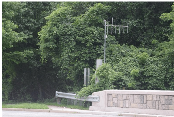
Typical Water Level Gauge Systems
